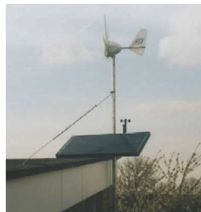
wind gen and PV: our installation at Tithe Farm School.
